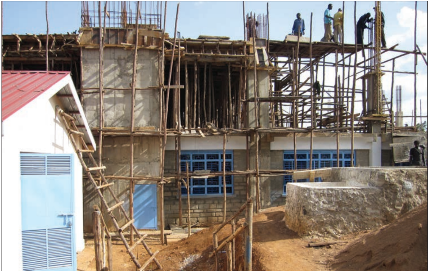
Tooth and nail: Workers construct the Moi University School of Dentistry's new building in Eldoret, Kenya.
